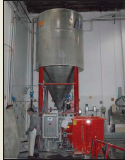
Silo where flocculation and particle separation occur. The red apparatus to the right is the filter press.
